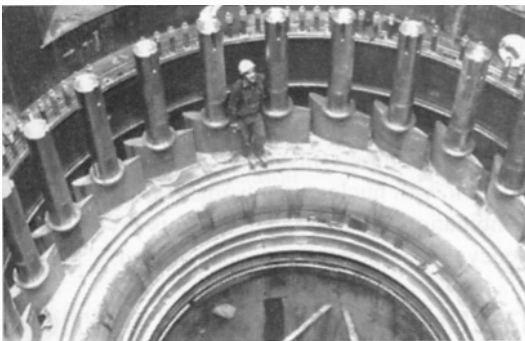
Figure 24.12 Inside the spiral case, a set of adjustable wicket gates control the amount of water flowing into the turbine. (Courtesy of Marine Industrie)
